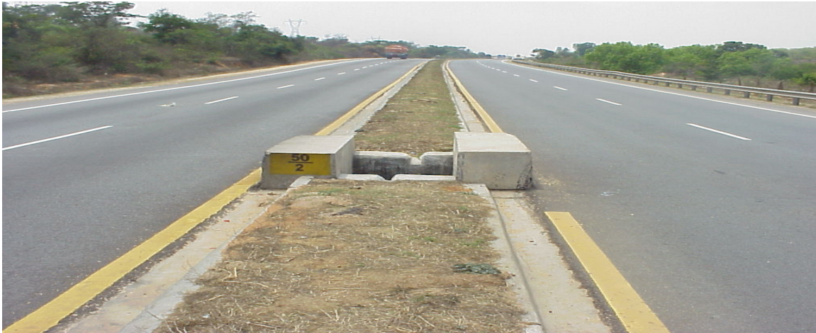
* Accident waiting to happen in NH-7 (note projecting structure portions)
